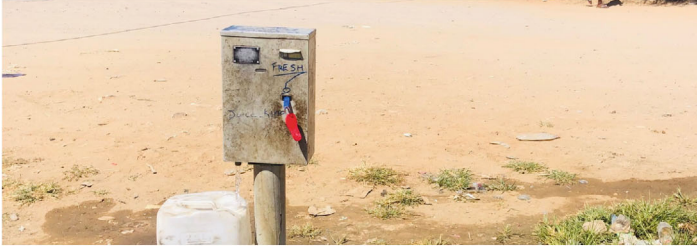
Frame b: Picture showing the provision of public water supply systems. A communal water tap in the Ekunde 2 informal settlement — ©Photograph by authors.
